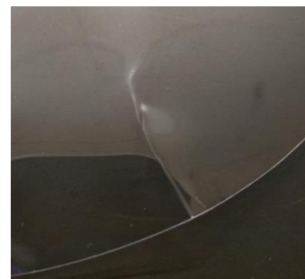
Figure 2: Creasing at corner.
